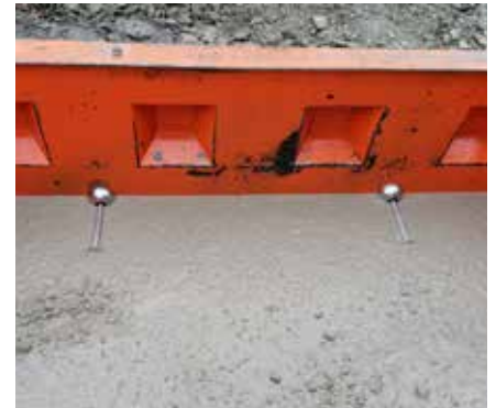
3 The anchor is cast in its entirety, be careful when vibrating the concrete.
